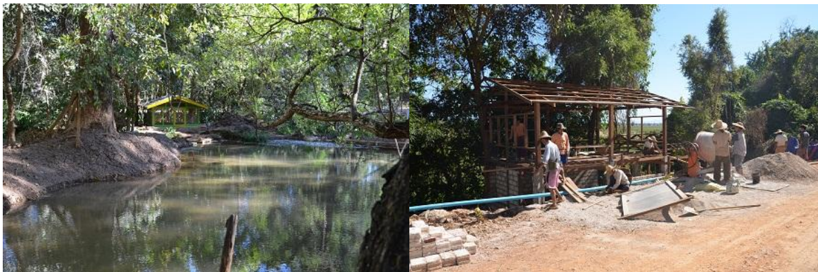
Figure 9 Ye U Water Spring and Construction of Water Pump House in Taungchay Spring for the development of water pipeline system
