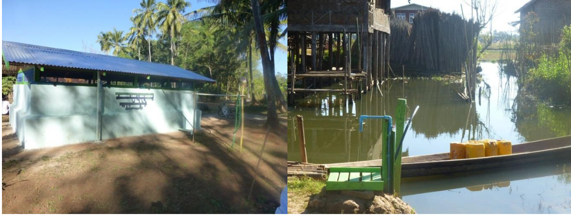
Figure 10 Complete construction of 3500 gallon tank and development of access to water by water pipeline system
