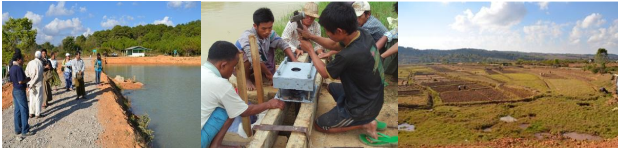
Figure 11 Renovation of sluice gate and weir of dam and newly irrigated farms
